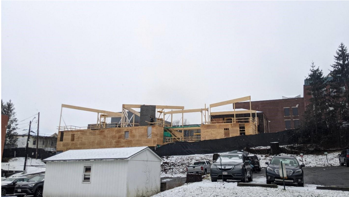
Construction of Williams College Davis Center, the first modern mass timber building in Williamstown.
