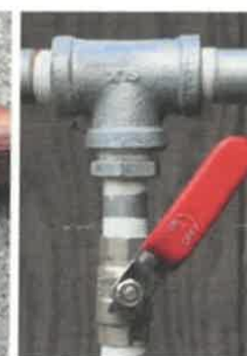
Galvanized Steel & valve
